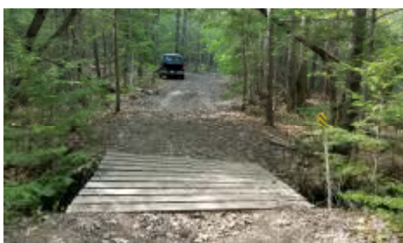
This bridge was built by volunteers of the local snowmobile club, the Cornish Snowcruisers. In addition to turning the road into a mud wallow, heavy vehicles had also broken down the support of one corner of the bridge.
